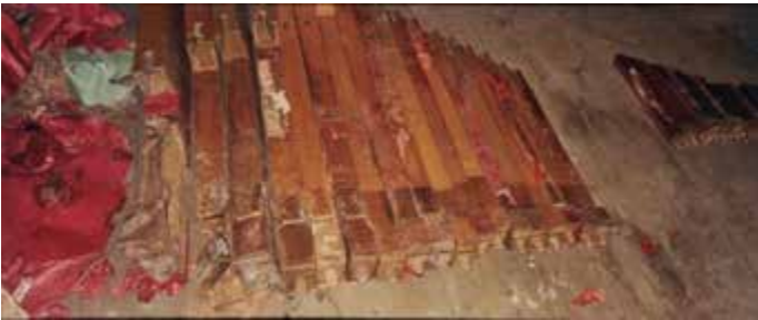
Fig. 3 Pipes rotted away from leaking roof
