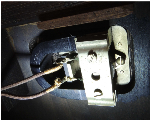
Fig 11: The transducer, mounted below the motor board.
